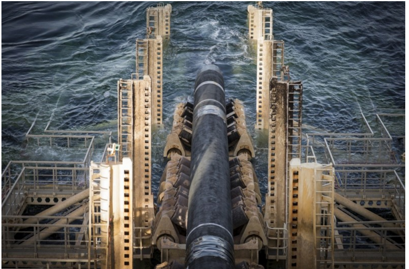
Nord Stream 2 pipe-laying in Swedish waters in the Baltic Sea. Photo by Axel Schmidt.
